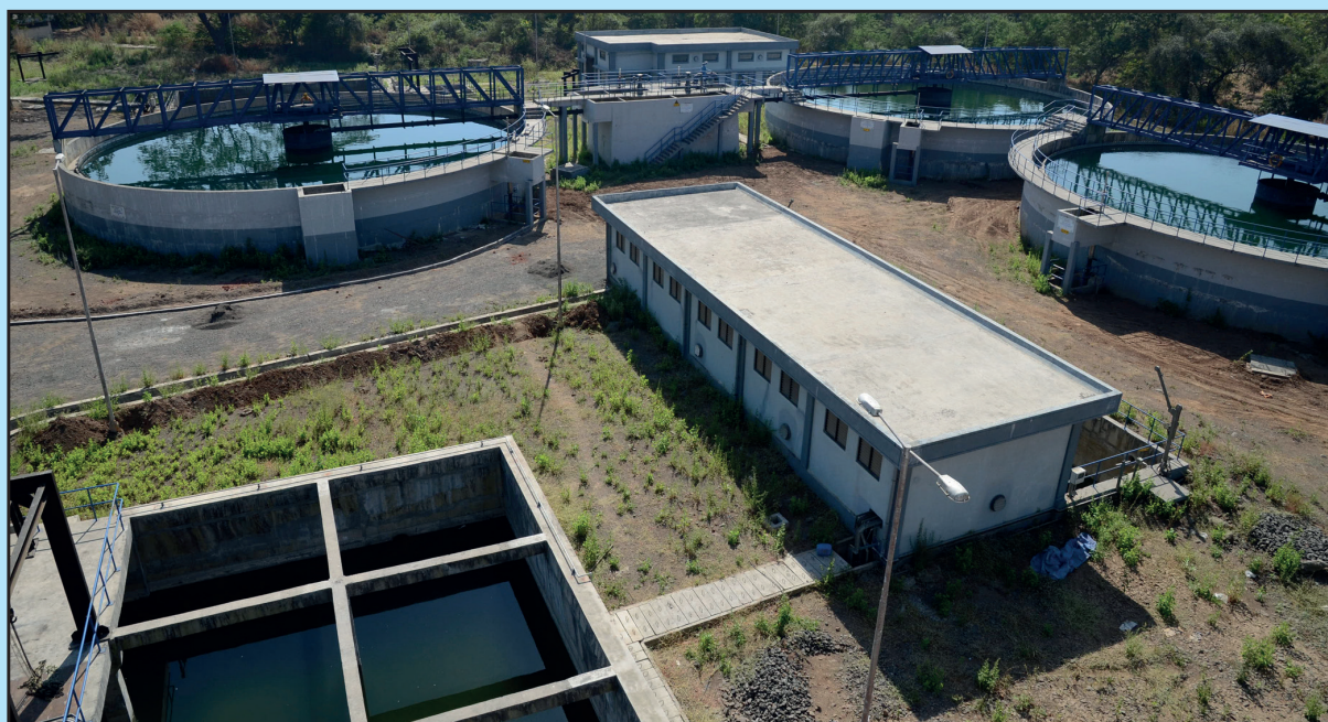
Membrane filtration plant at Bhandup Complex
